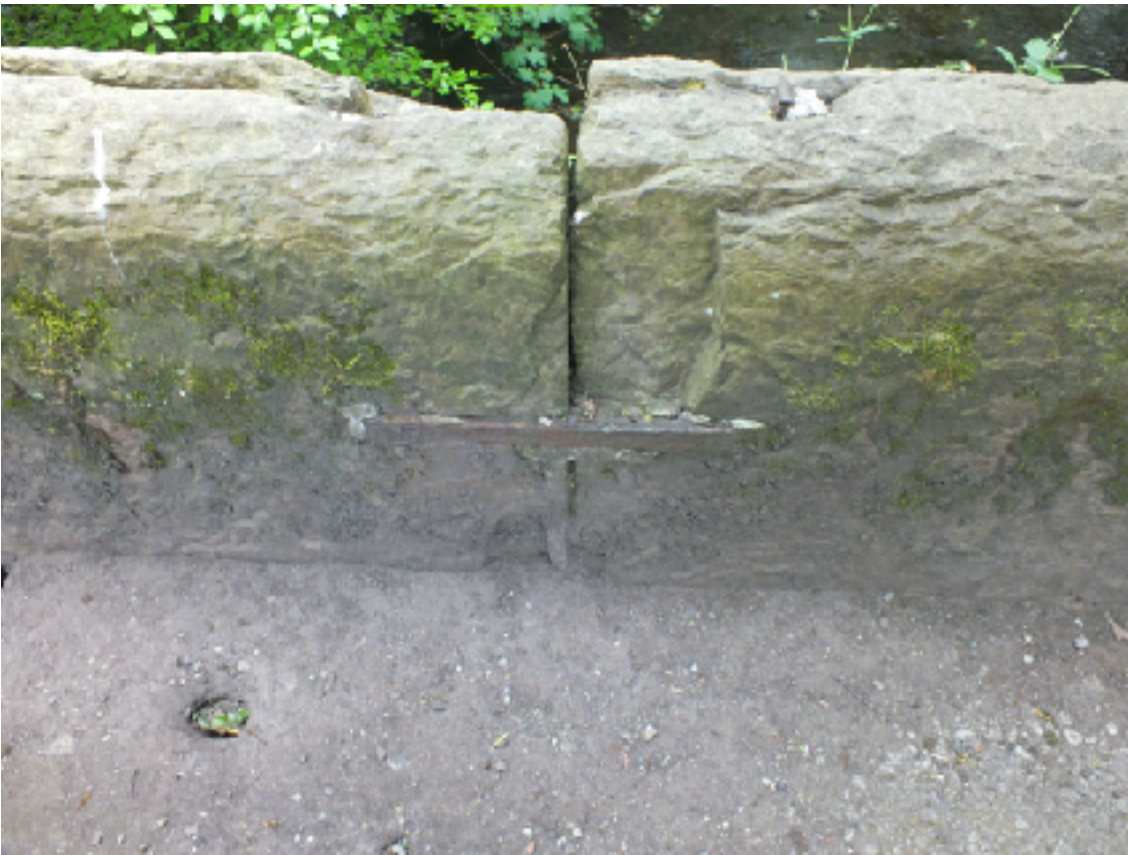
Image 5. The parapet stones were also held by horizontal steel bars. This one is still holding whereas the top steel had gone, just a small piece of steel is on the right hand side.
