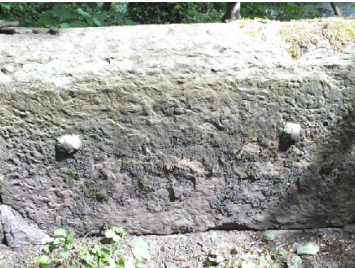
Image 6 Lane side of a spit parapet stone on the upstream side held together with two bolts Hoggs Lane bridge, need for maintenance
